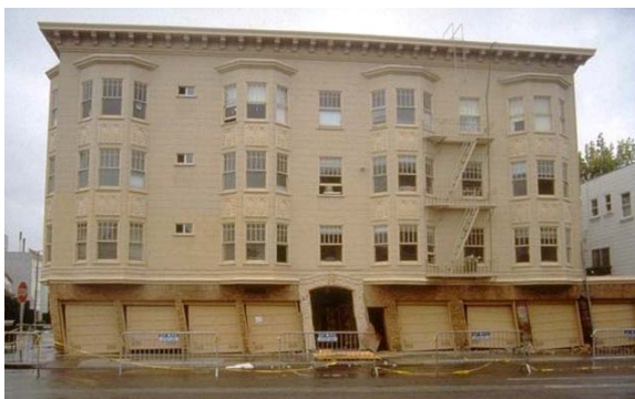
(e) Loma Prieta building damage.
